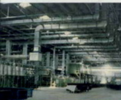
AIR DUCT & EXHAUST SYSTEM
